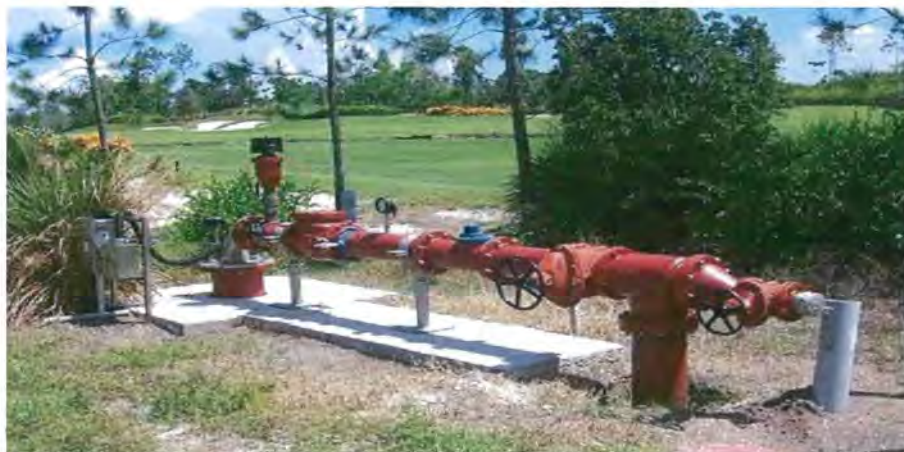
Photo 4: Surficial Aquifer Well
